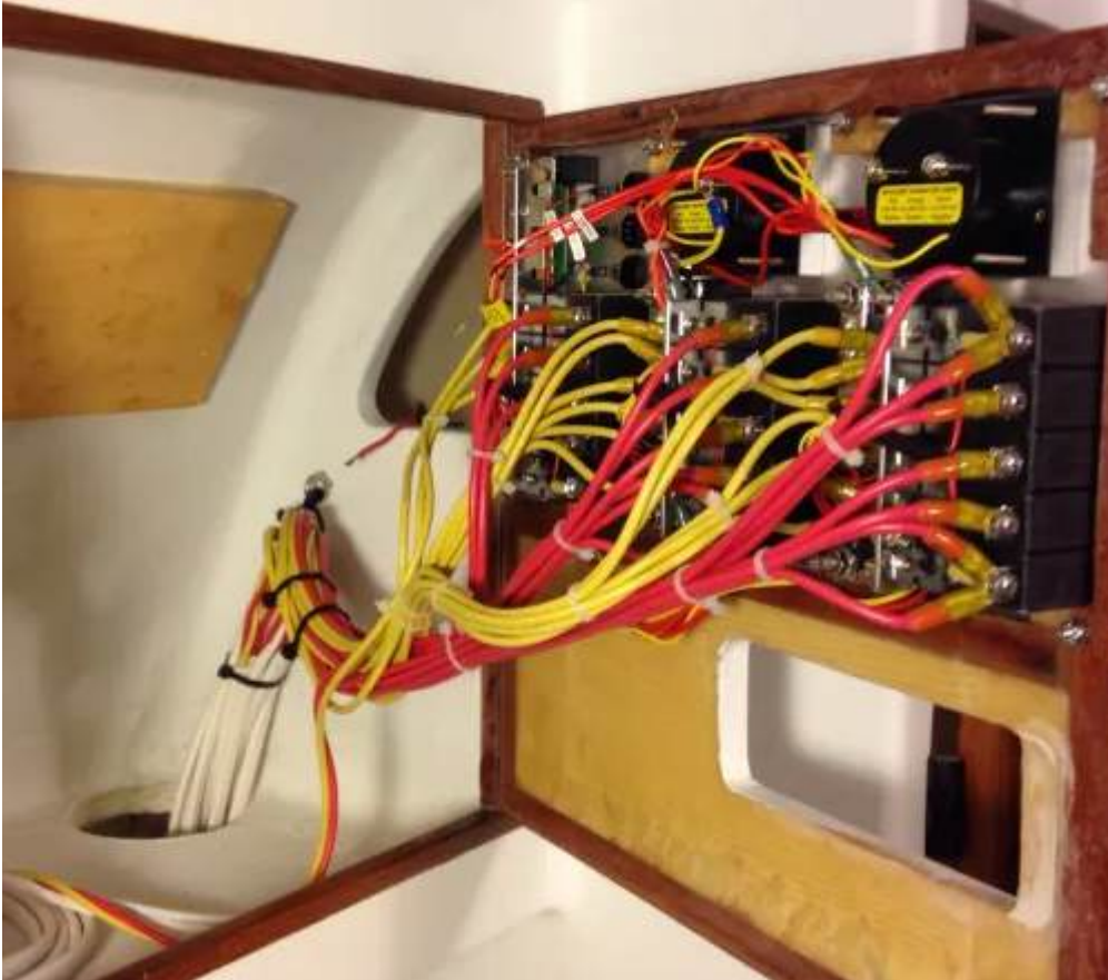
Photo: a typical small vessel DC panel, post 2008.
